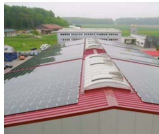
Industrial construction DE Built in 2009 Power 105 kWp
